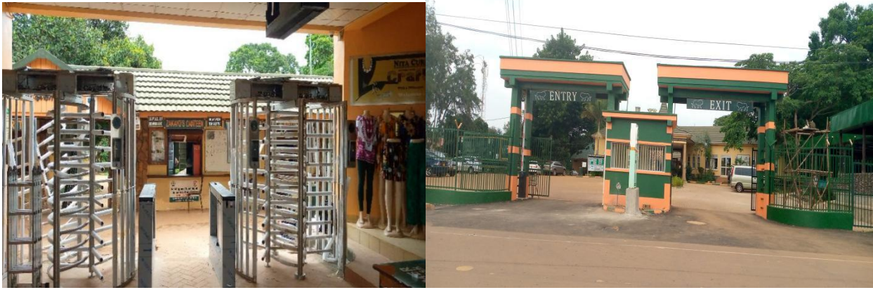
Electronic access control system and gate installed
