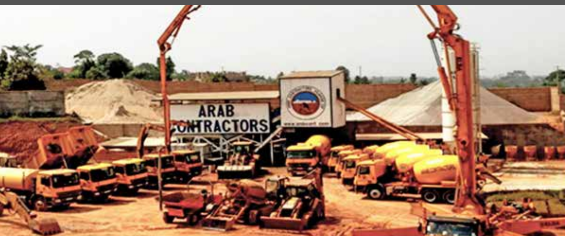
Arab Contractors Batch Plant
